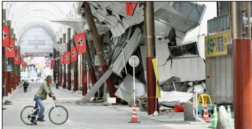
Shopping arcade collapsed
